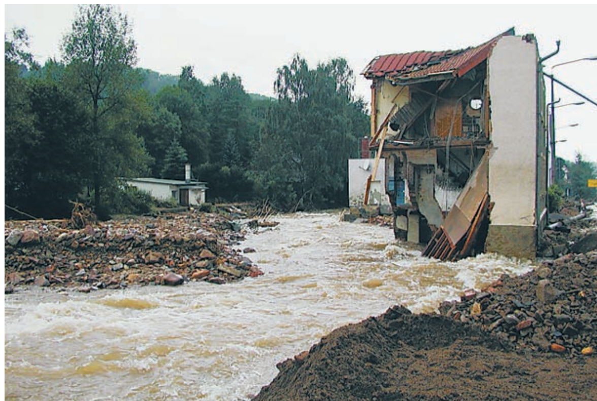
Fig. 8: Destroyed building and channel displacement of the Rote Weißeritz in Schmiedeberg (photo: GOTTFRIED HEROLD, 2002)
